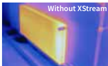
Radiator with trapped air at the top and dirt blockages at bottom
